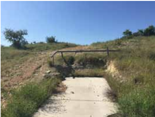
Exterior - Damaged Concrete Path
